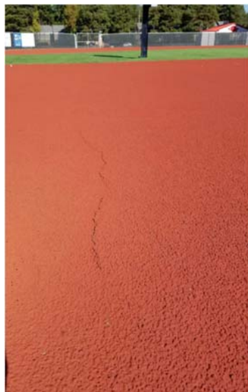
Example of a surface crack
