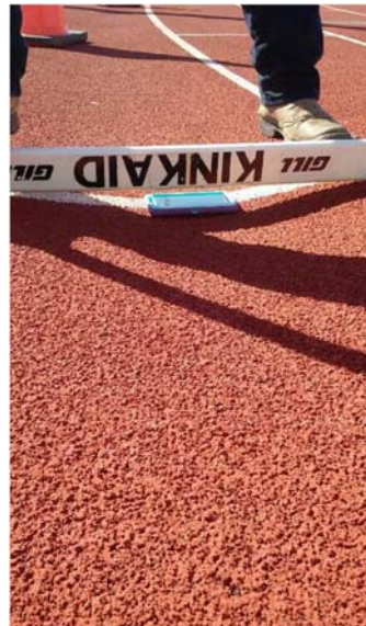
Example of a dip in the track surface. This would be a problem below the subbase.
