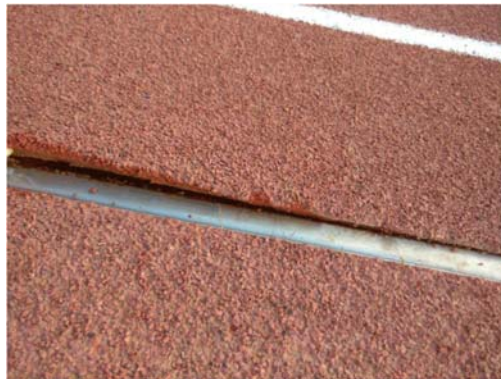
This is a delamination, where the top track surfaces is separating from the asphalt base.
